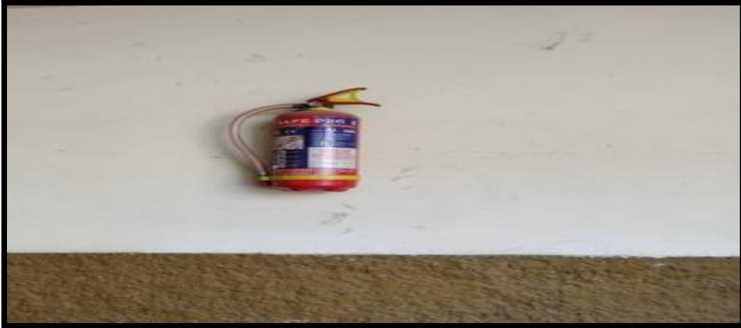
Fire Extinguisher (at different places)
